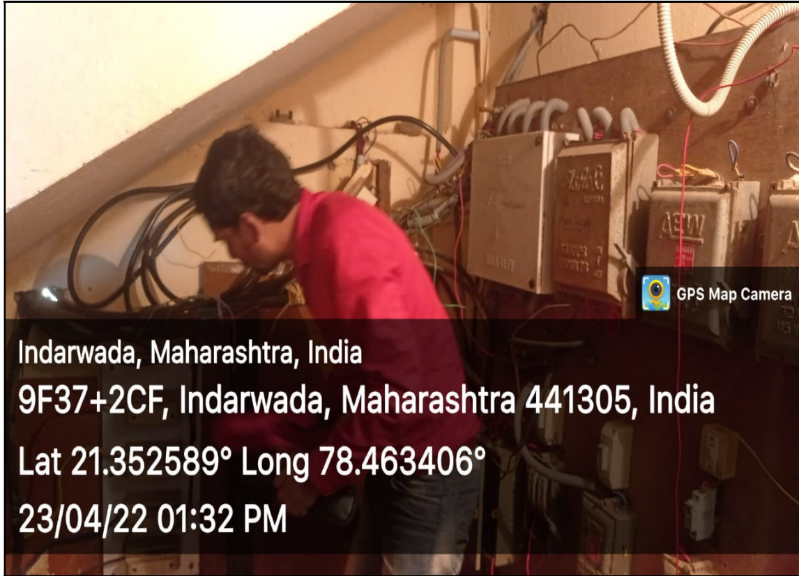
Fig.-4.2 Photograph of ON Site power measurement in college campus
