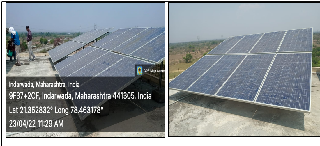
Figure 2.1: Solar Power Plant 10 KWp
