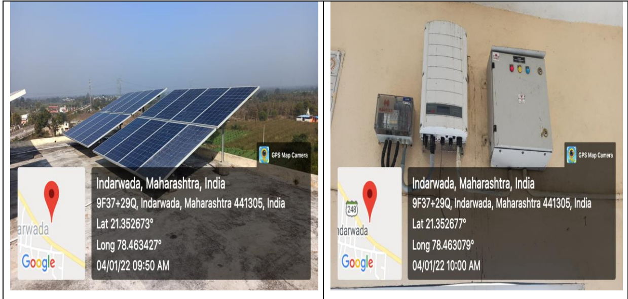
10 KWp solar plant and Inverter systems.
