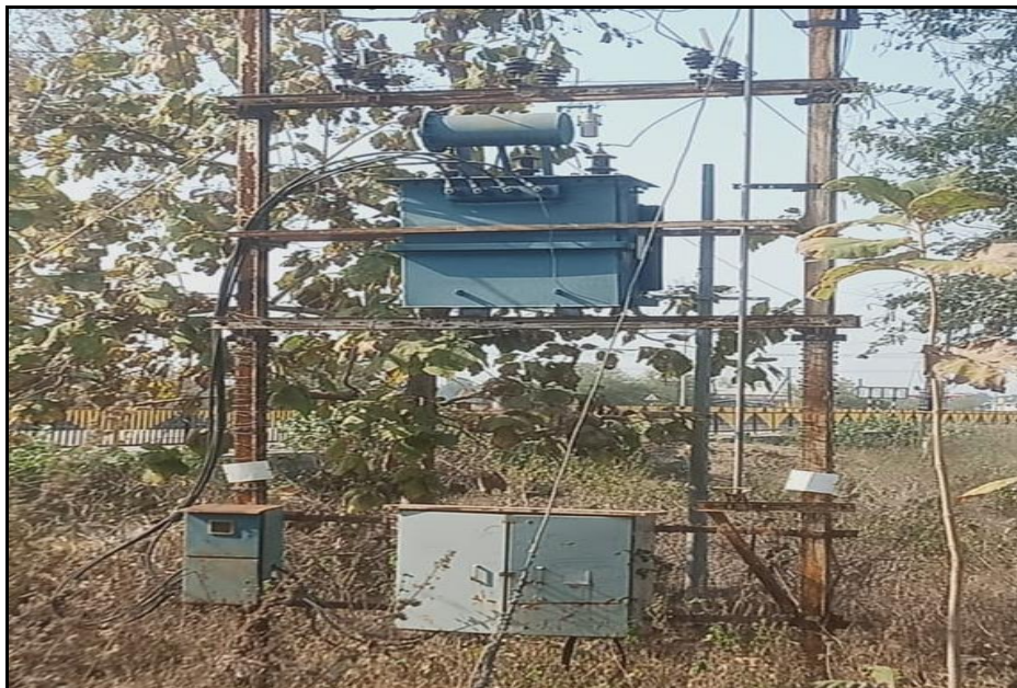
Photograph of transformer
