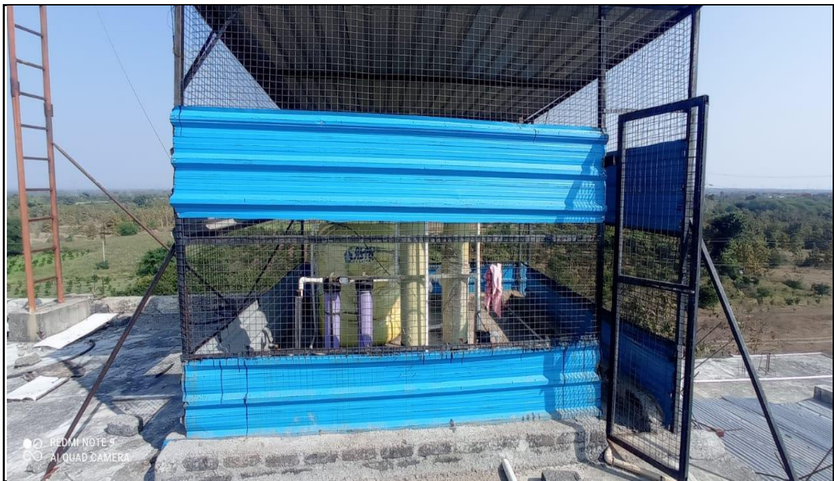
RO plant in college campus
