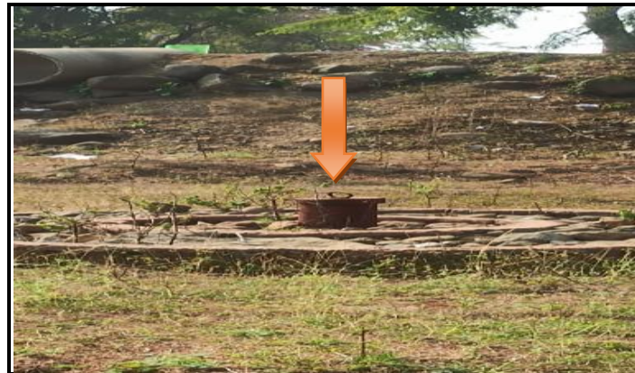
Fig:- 2.3 Requirement of water meter on bore well
